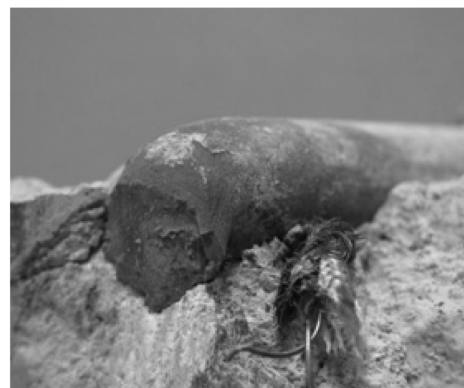
(b) Failure of headed stud
